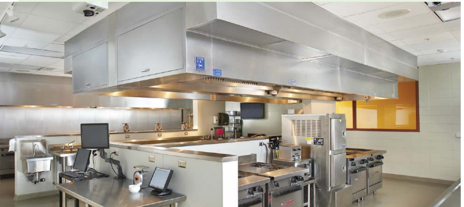
Photo Courtesy of Greenheck Fan Corporation
