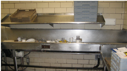
NO SUPPORT STRUCTURE
